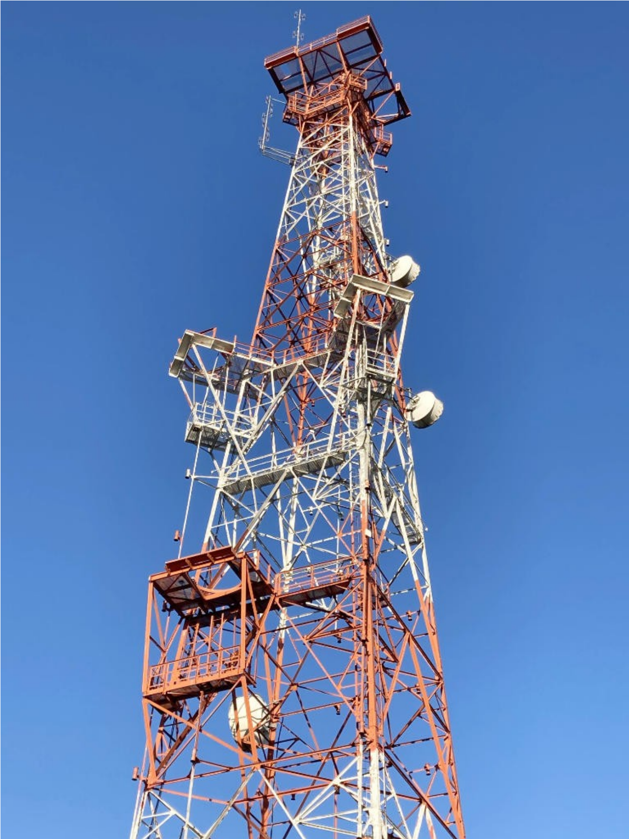
Tower with two dipole array antennas and three shrouded parabolic antennas.
